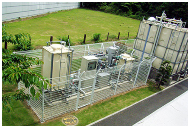
Decentralized water treatment & supply system
