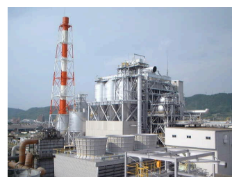
Biomass boiler at the Hiroshima Plant
