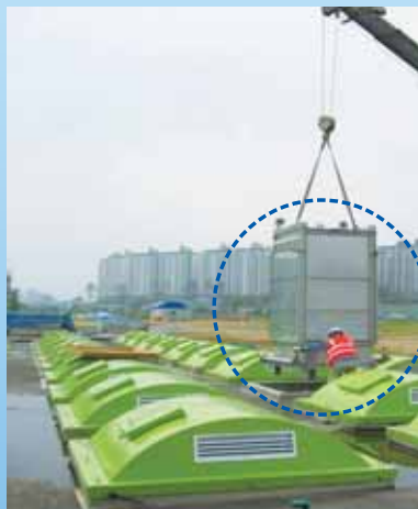
The "STERAPORE" hollow-fiber membrane filter is installed in a wastewater treatment facility.
